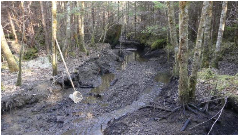
Figure 8. A section of formerly ponded channel about 70 feet downstream of the highway. View looking upstream.
