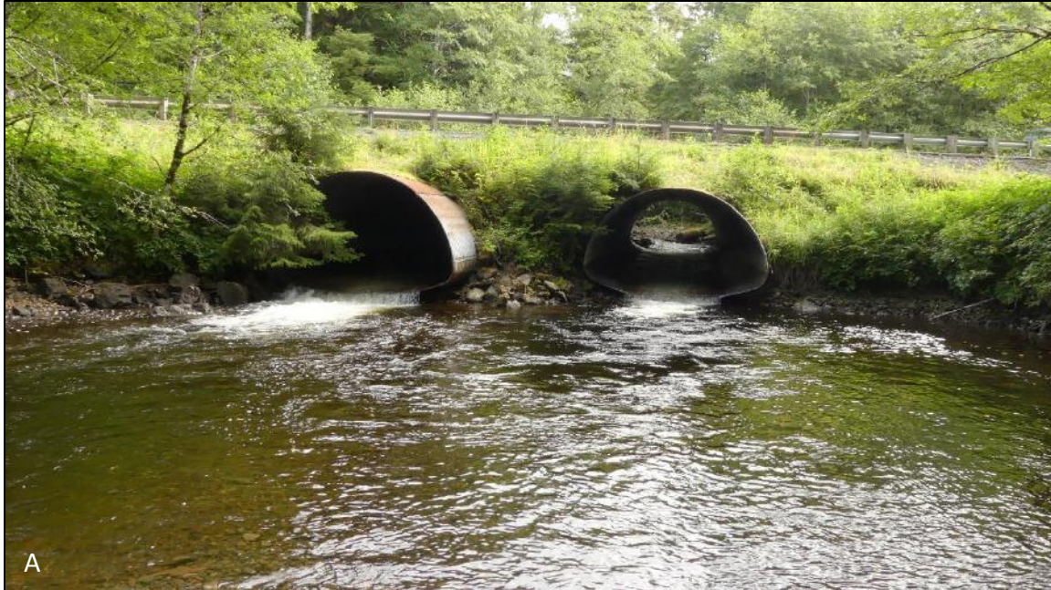
Figure 5. (A) Low flow through the double culvert at the Klawock-Hollis Highway crossing August, 2018. (B) Illegal cutting of large woody debris in the channel immediately downstream of the highway. (C) Downstream end of the sediment slug where sediment aggradation has caused channel avulsion and raised the water resulting in tree death.
