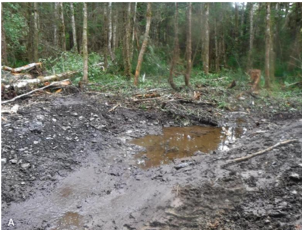
Figure 2. From the Pat Creek Fish Habitat Enhancement Project. (A) Example of a road breach excavated to the elevation of the surrounding grade on an alluvial fan. (B) Schematic of a typical road breach. (C) A logging road on an alluvial fan after removing alder trees to access breach sites.
